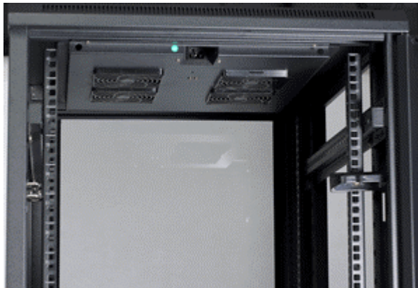
Four ball bearing exhaust air fans at the top.
